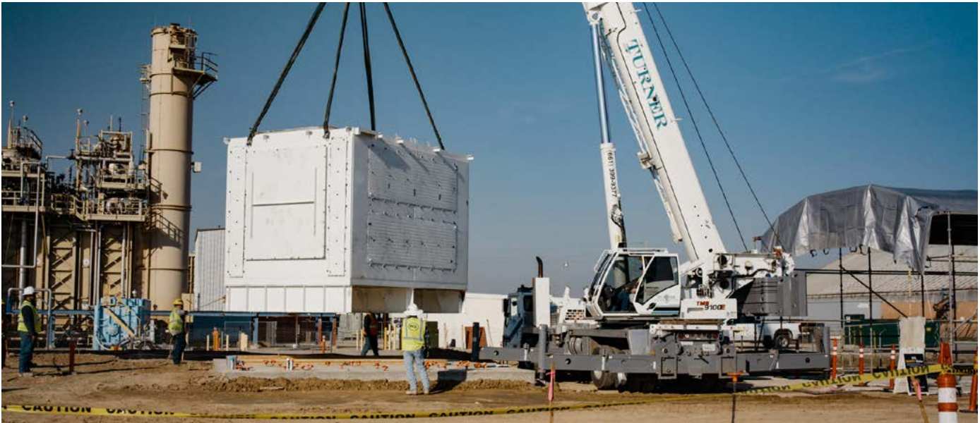
Antora Energy has developed a low-cost, highly efficient thermal battery that stores electricity produced by wind and solar generators as heat, allowing manufacturers and other energy-hungry businesses to eliminate their use of fossil fuels. Above: Antora installs its first commercial-scale unit at an industrial site near Fresno, California. Photo courtesy of Antora Energy
