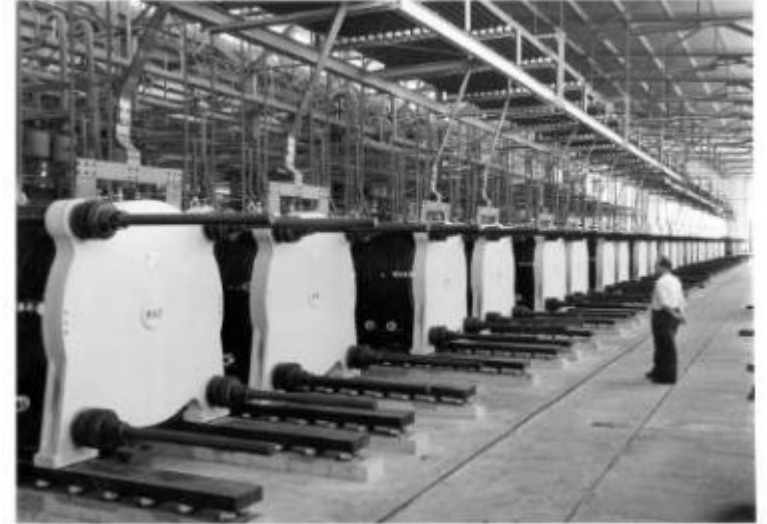
135 MW KOH plant: 257,000,000 cm 2 10,000,000x test cell
