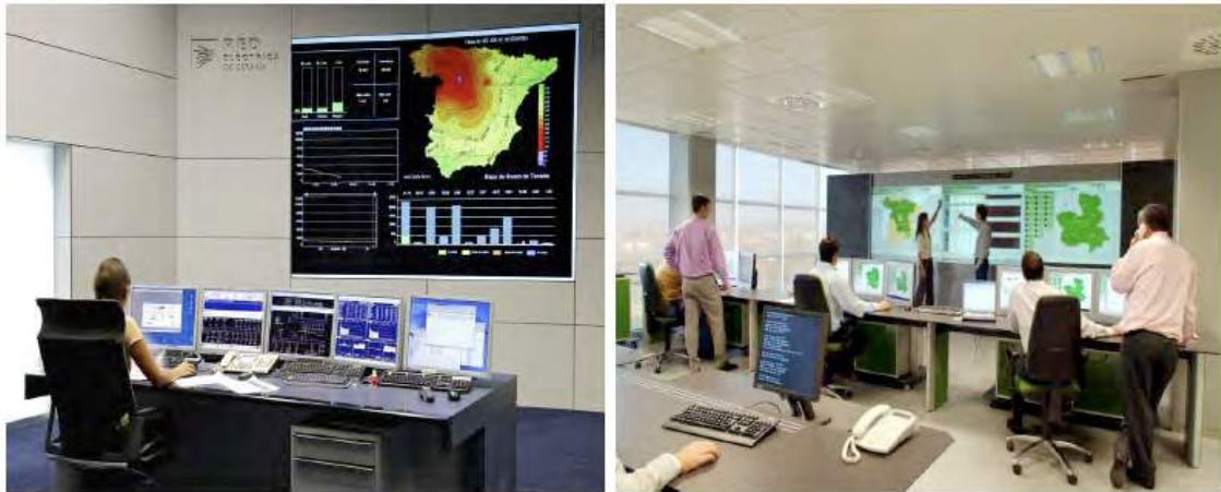
Figure 14: National control center for renewable energies in Red Eléctrica, the Spanish system operator (left) and Iberdrola's wind control center (right), one of the 14 satellite control centers for wind in Spain.
