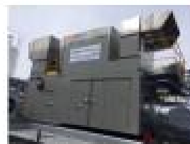
Hydrogen Gas Turbine (1MW class)
